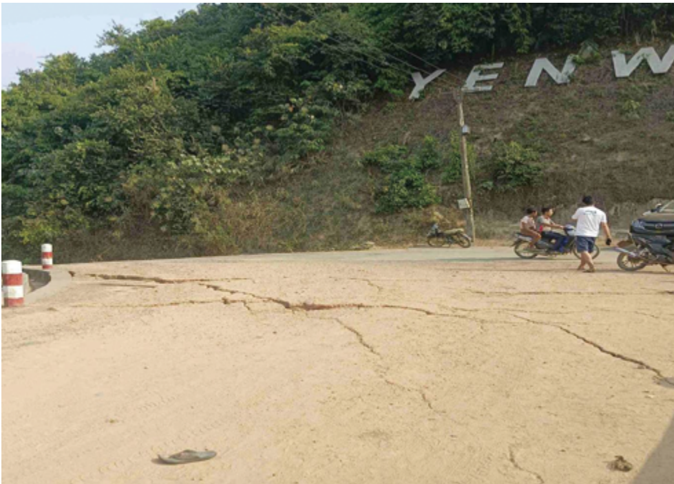
Fig. 12: Ye Nwe Dam Crack Line at the Right Abutment
