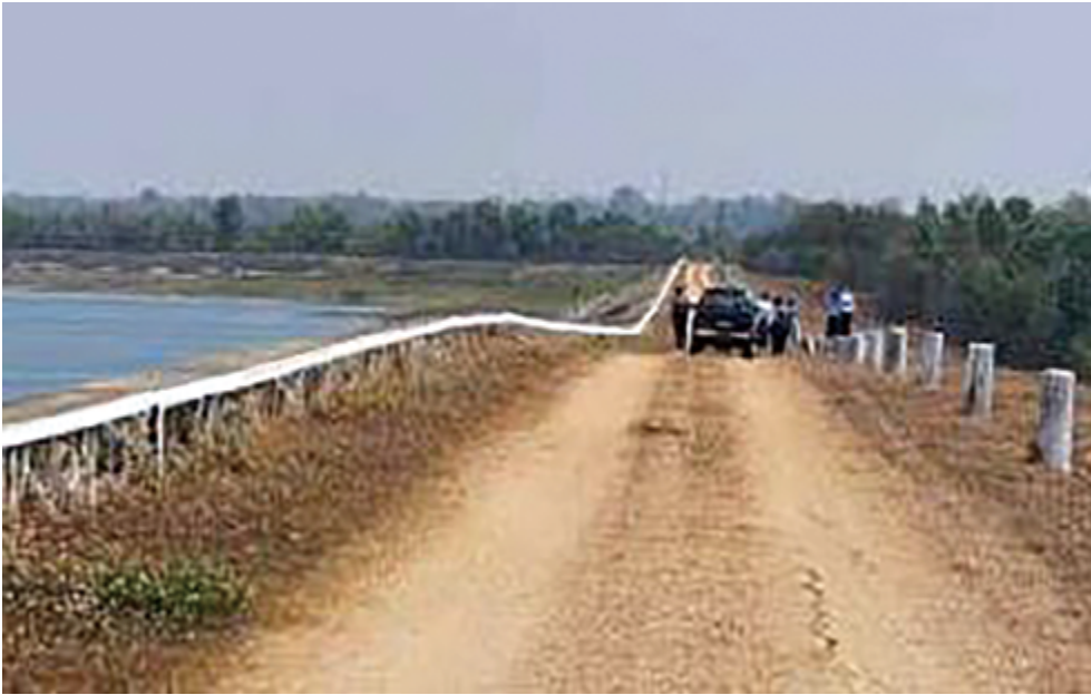
Fig. 16: Chaungmagyi Dam Differential Settlement of Dam Crest at R.D 5000 ft
