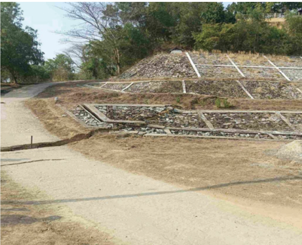
Fig. 11: Ye Nwe Dam Crack Line at the Left Abutment
