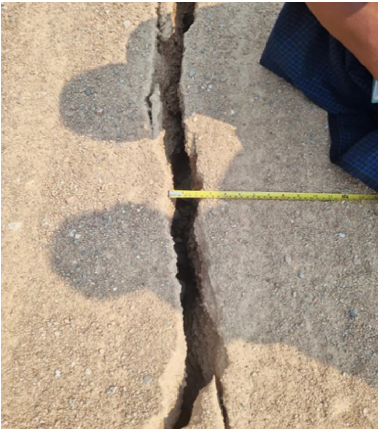
Fig. 14: Lower Paunglaung Dam Measuring Width of Crack Line
