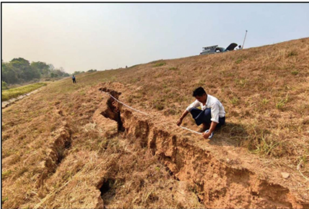
Fig. 17: Chaungmagyi Dam Longitudinal Crack Line on the Dam Downstream Face at R.D 4200 ft
