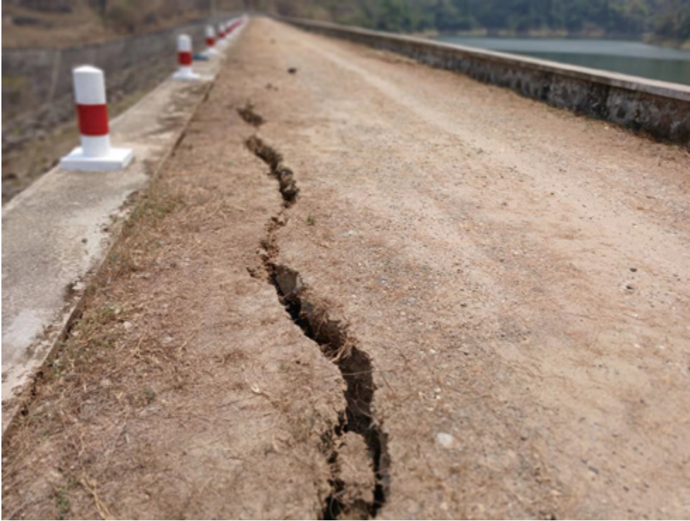
Fig. 9: Phyu Chaung Dam Longitudinal Crack on the Dam Crest (R.D 700 ft)
