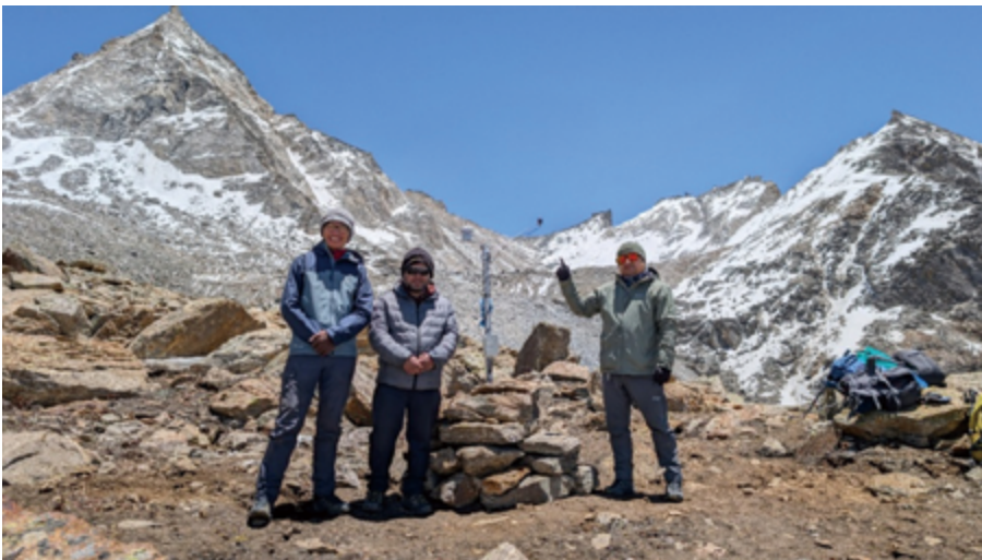
Figure 19: Micro-weather station installed near the lake drained area at 5,270 m asl, measuring relative humidity, air temperature, solar radiation, soil moisture, and soil temperature from 20 cm below ground up to 2 m above the surface in stable terrain.
