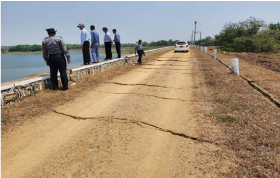
Fig. 15: Chaungmagyi Dam Transverse Crack Lines at R.D 3800 ft
