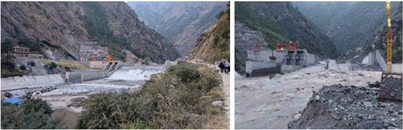
Figure 23: Before (November, 2024) and after (9 July 2025) photographs showing the Hydropower dam was completely collapse. (Photo by Sudan Bikash Maharjan (left) and online sources (right).)
