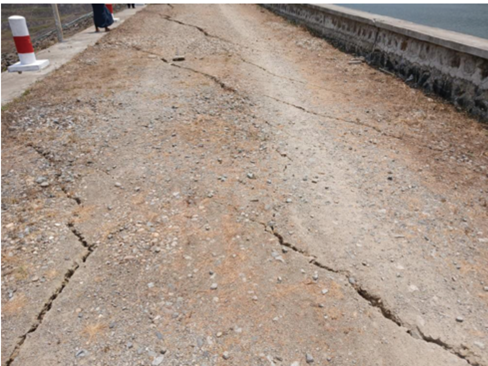
Fig. 10: Phyu Chaung Dam Diagonal cracks at the Dam Left End (R.D 50 ft)
