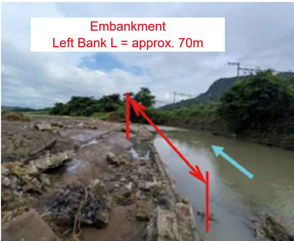
Figure 14. Restoration Works for the Kiba River within the Kikuchi River System (Tamato Town, Kumamoto Prefecture)
