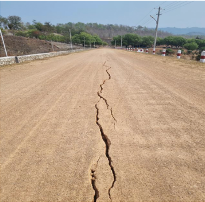
Fig. 13: Lower Paunglaung Dam Longitudinal Crack on the Dam Crest
