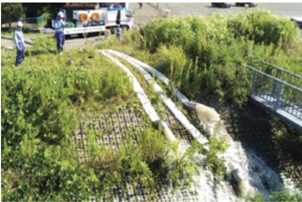
Figure 15. Drainage Support Using Drainage Pump Vehicles for Inland Water Removal (Kanagawa City, Ishikawa Prefecture)
