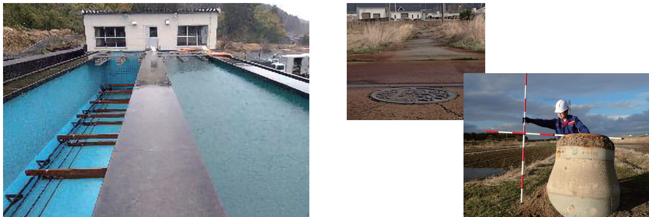
Figure 2. Damage with and without earthquake-proofing (left: water treatment plant; right: utility holes floating up)
