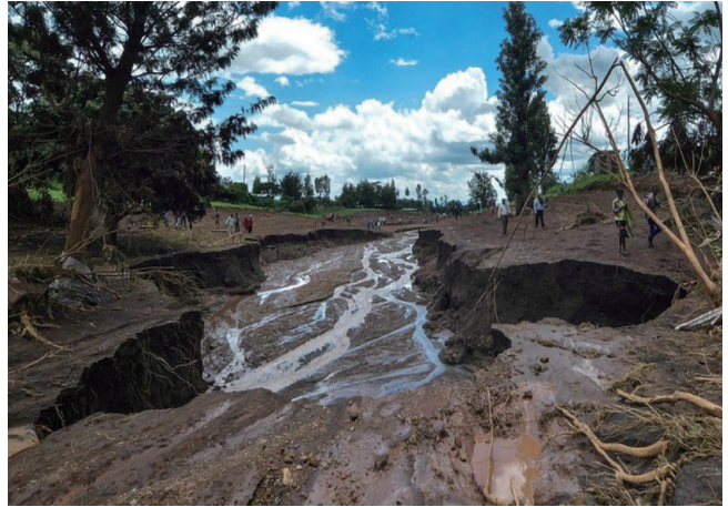
Figure 14: Water curved fissure from Patel dam burst
