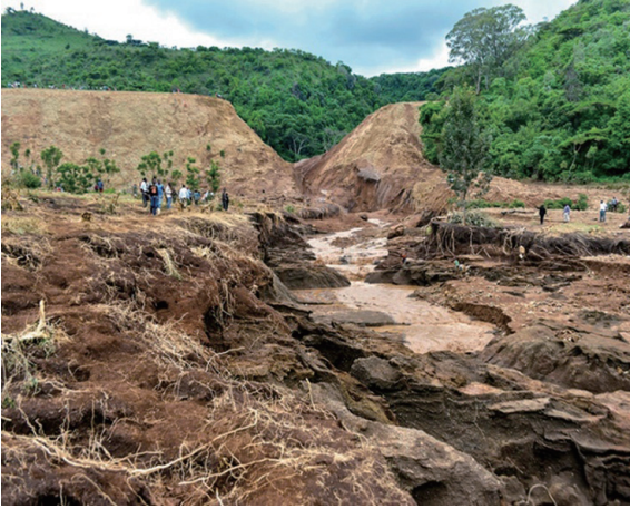
Figure 10: Breached section of Solai Dam
