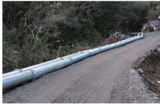
Figure 6. Temporary Piping (example of using rolling piping)
