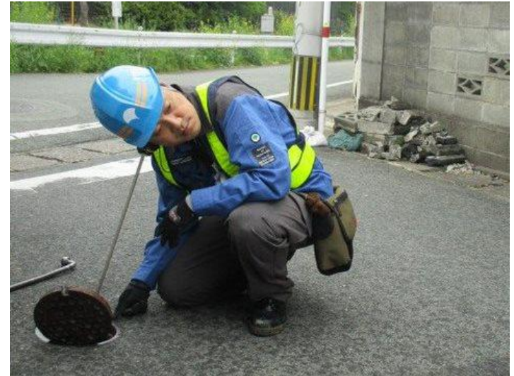
Inspection of Water Leakage (from website of Tokyo Metro. Gov.)
